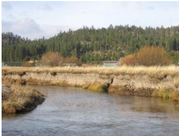
Extensive erosion is evident along the banks of the Upper Truckee River in the area near the Airport runway
